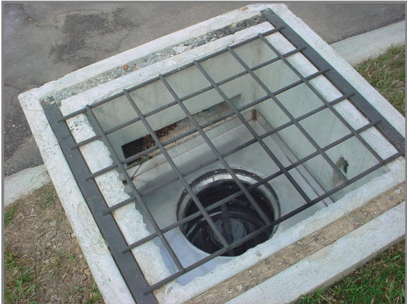
The surface grate over an Aqua-Guardian™ unit
